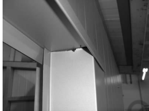
The window reveal plate is fitted behind the drip profile. Behind that is the Type 8 vapour permeable sealing tape. A soffit lining made from an edge-folded plate is suspended from the front edge and attached to the window at the back.
