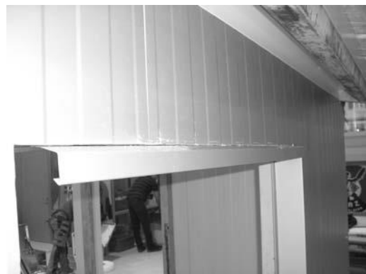
The best sealing is achieved through the correct use of sealing tapes combined with the craftsmanship of the sheet metalwork. Drip profile installed the panel.
