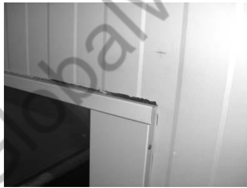
The reveal cladding sheets are nested at high level. With this method it is important that Type 8 window sealing tape is carefully applied under the cill profile and reveal cladding sheets without puncturing.
