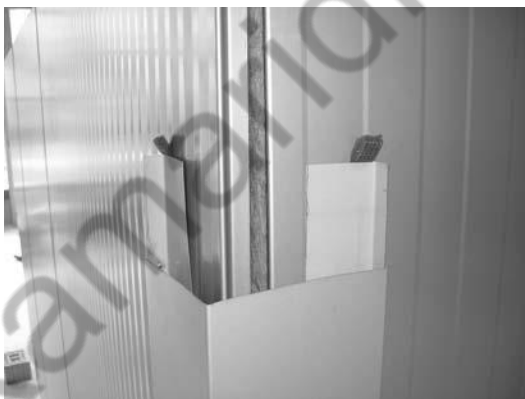
The more elegant corner detail using a concealed support angle. A Type 4 sealing tape must be installed between the panel surface and the support angle. The fastening brackets can be fitted using self-drilling screws. The corner cladding itself is fastened to the sides of the support angles using coated aluminium rivets with a stainless steel mandrel.
