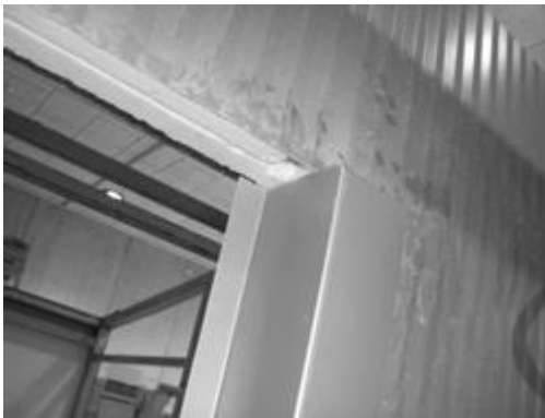
The foam on the lintel behind the outer seam is removed to form a slot for the later installation of the vertical seal. A recess must be made in the foam on both sides above the window reveals to provide space for raising the upstand profile.
