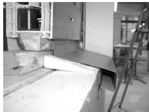
The correct installation of the cill profile. The windows must be fitted with a suspended cill profile. The fall on the cill to the outside must be at least 3° with a projection of at least 25 mm. The vertical face dimension must be not less than 20 mm.
